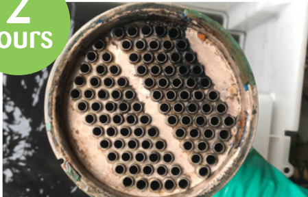
Volvo Heat Exchanger after 2 hour treatment of CleanScale.
